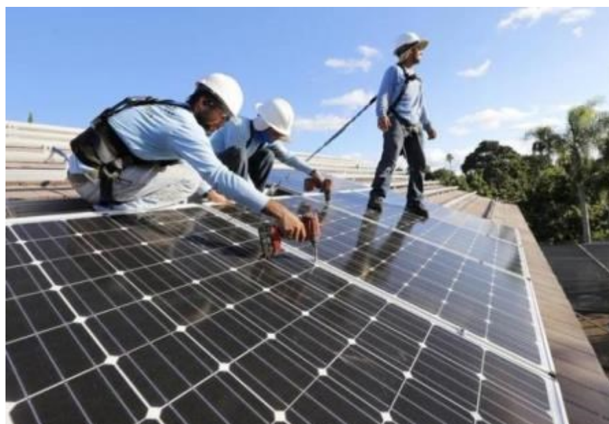
Figure 4 – Example of installation of a PV System in the presence of several risks
